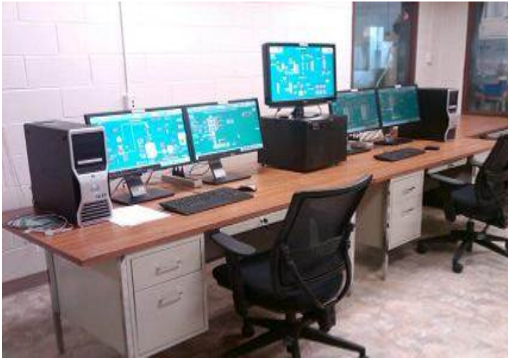
Figure 26—IH 2 Control Room
